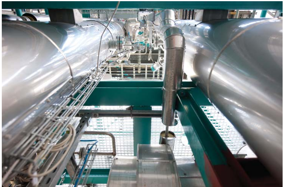
The absorber and desorber columns at the Staudinger pilot plant in Germany. Source: Siemens/E.ON
